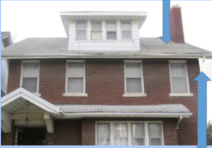
Missing Downspouts and gutters in poor condition
